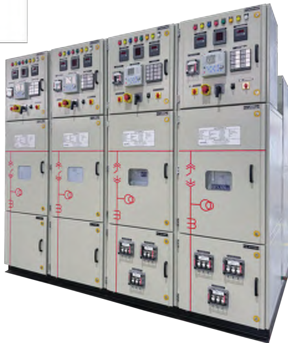
38kV Metal-Clad Medium Voltage Switchgear
